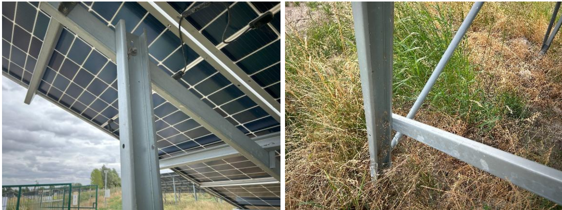
Plate 12-15 Indicative thin racking system driven into ground
